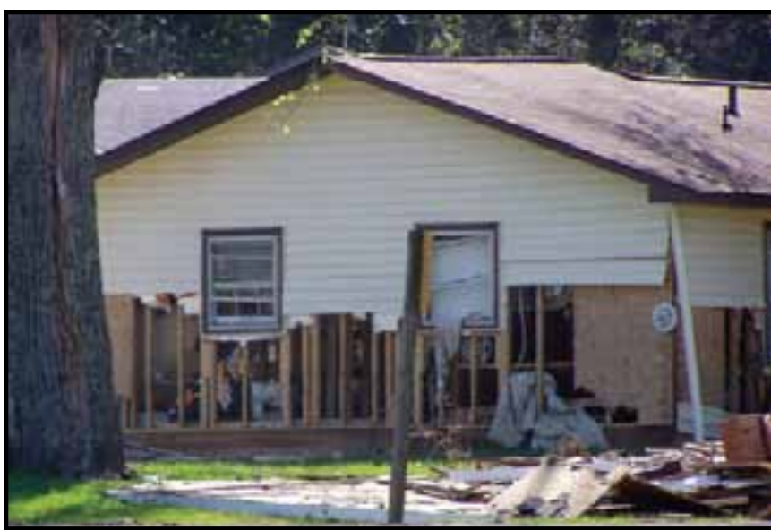
A structure damaged by a Hurricane.
